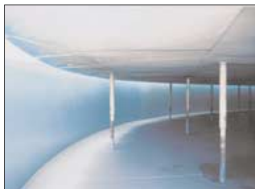
Fig. 3 - Underside of a 140-foot (43-meter) floating roof tank lined with a 50- to 60-mil (1- to 1.5-millimeter) AHC epoxy for sour service Courtesy of Industrial Environmental Coatings Corp.
